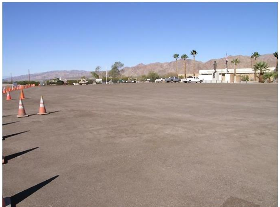
A photo of DACE/RANCHO's renovation of the Gen. Patton Memorial Museum parking lot, taken on Nov. 14 by RANCHO Project Manager Katherine Mejia. The $30,000 resurfacing was performed by One General Engineering.
